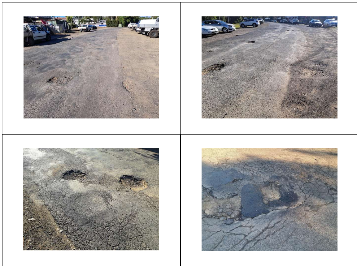
Figure 5: River Terrace Pavement Condition [2]
