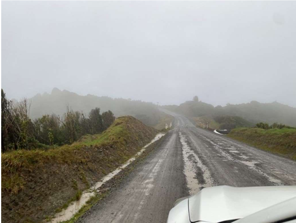
Pavement Rutting On a Gentle Graded Access Track
