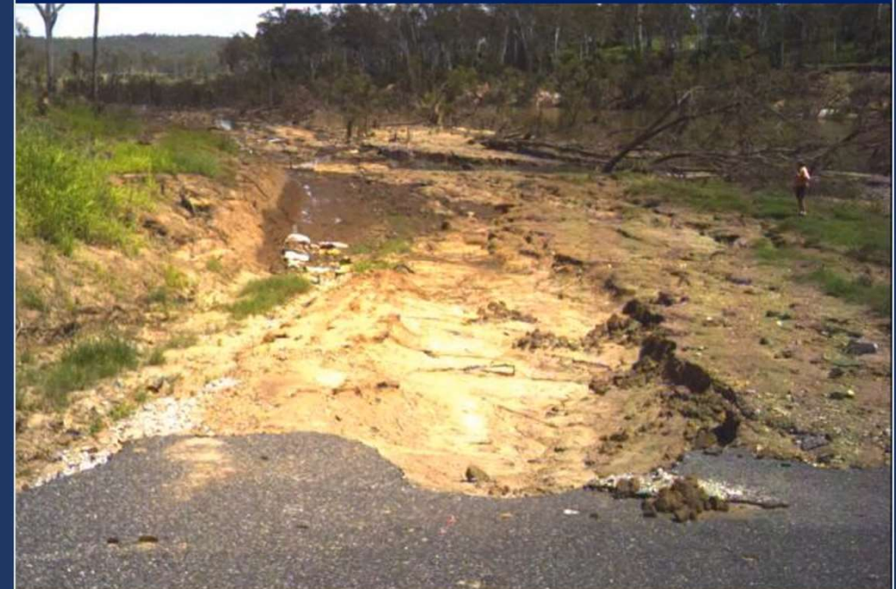
Gayndah Mundubbera Road damage following Cyclone Oswald 2013
