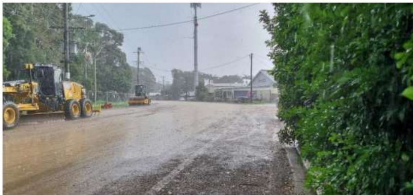
Figure 18: Wet Weather Prior to Sealing
