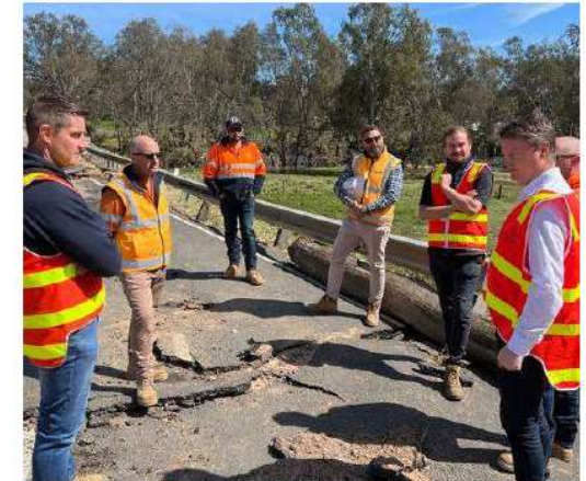
Roads Minister Ben Carroll (right) examines damage to the McIvor Highway, Axedale. Picture supplied by the Department of Transport.
