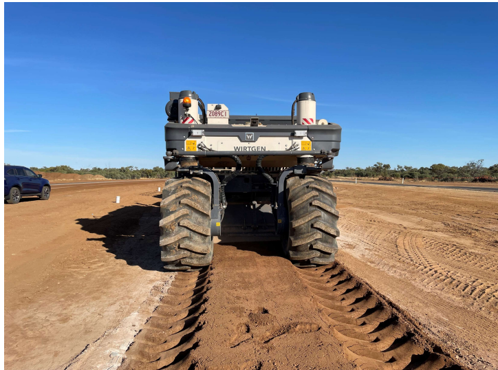
Sample taken directly behind the stabiliser
