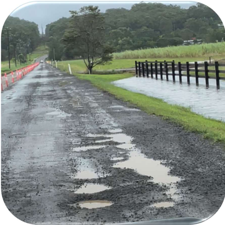
After flooding - untreated section
