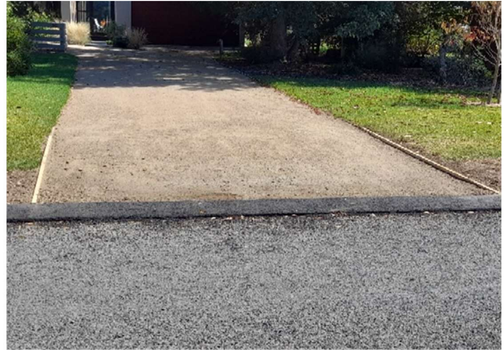
New kerb finished with layback making it easier for people to use their driveway
