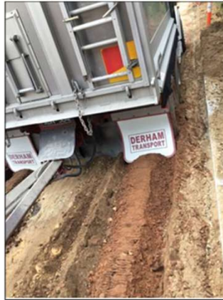
Struggling to keep the subgrade trafficable
