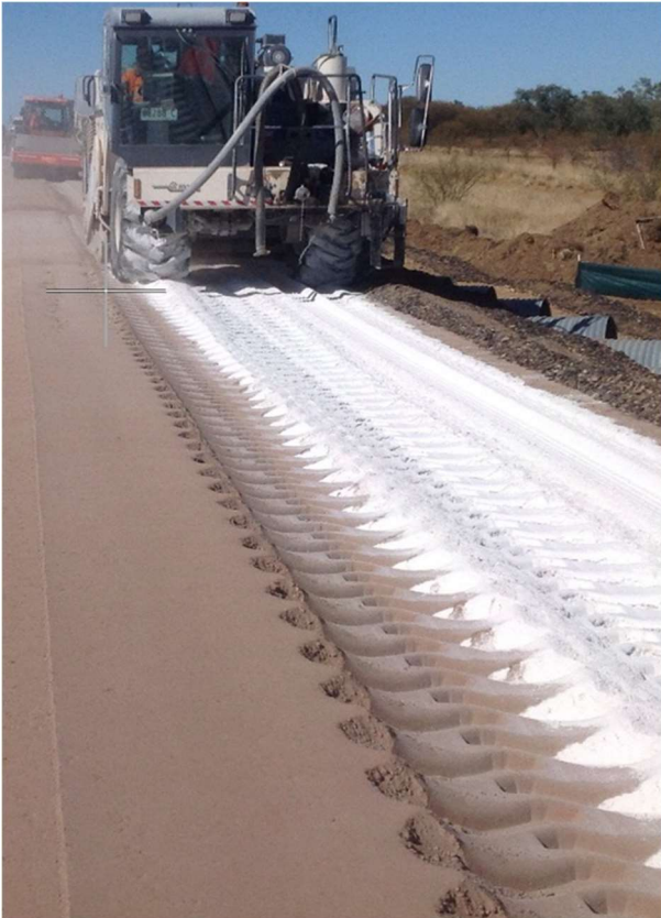
Triple blend dry powder binder in place prior to in situ mixing by a stabiliser
